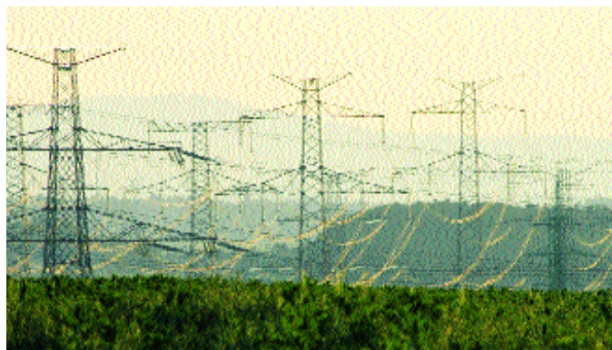
ČEPS transmission system
