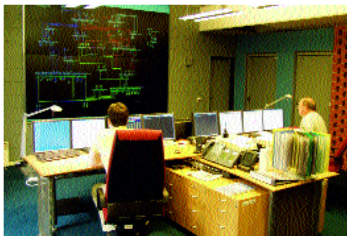
PRE control hall
