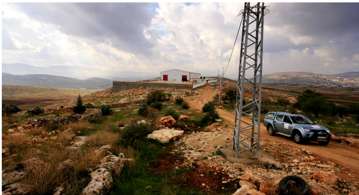
Palestine: Servicing station for transformers in Tubas
