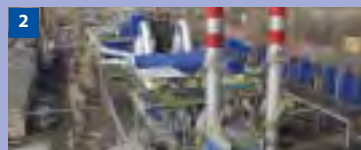
FOTO 1 – ESPs EKG, dedusting of 4 dry-bottom boilers for lignite combustion, 4 x 547 t/h, 4 x 220 MWe, ČEZ a.s. - Tušimice Power Plant, CZ
